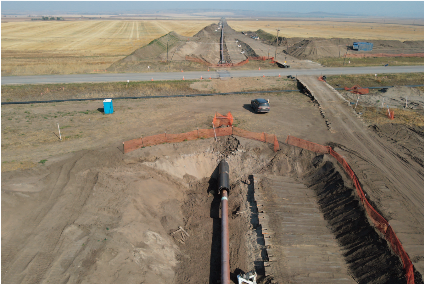
Figure 3. If a road can't be closed, why not go under it? Having straight open workspace to accommodate a single pull section is increasingly rare
